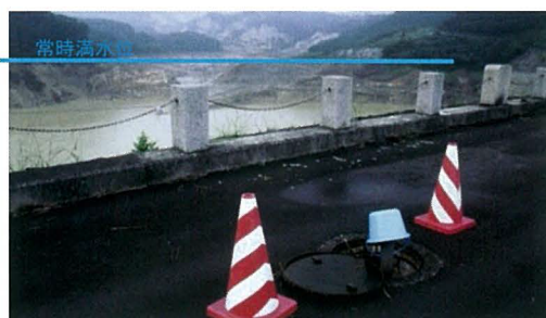
Fig. 22 堤頂での変状 Damage at the dam crest of Aratozawa Dam
